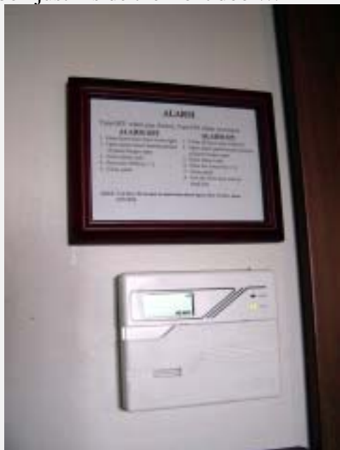
Alarm box just inside the front door...
